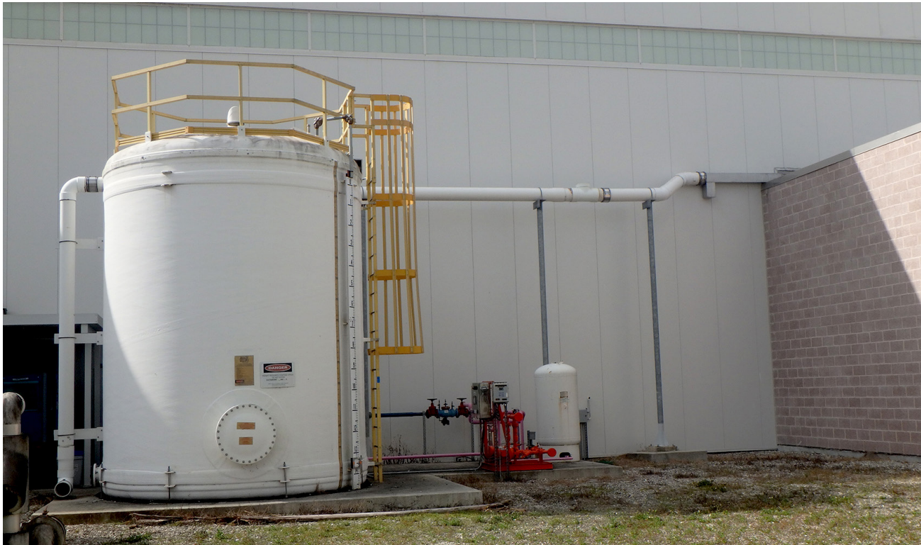
Rainwater harvesting tank.
