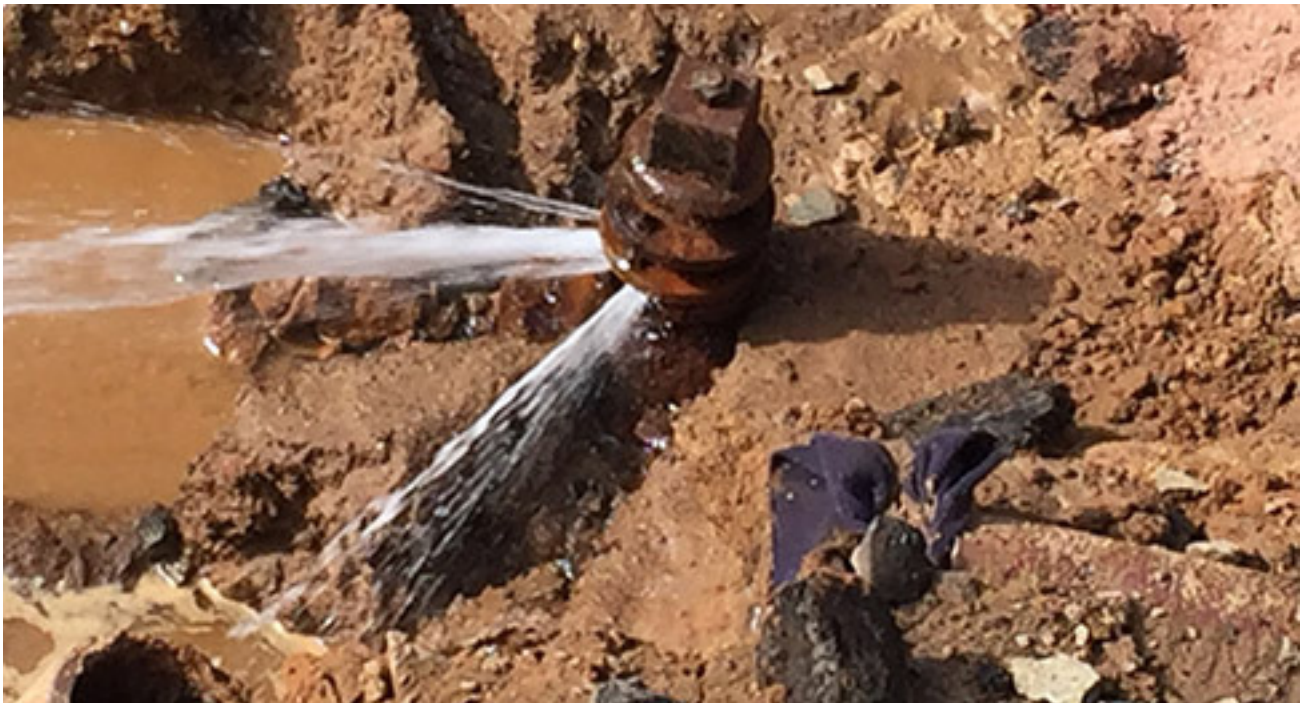
A sudden increase in water use is an indication of a potential leak.
