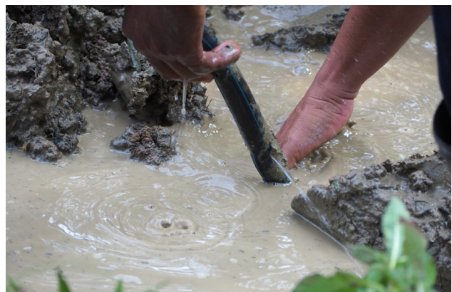
Wet areas above an underground pipe can be an indication of a broken pipe or joint.
