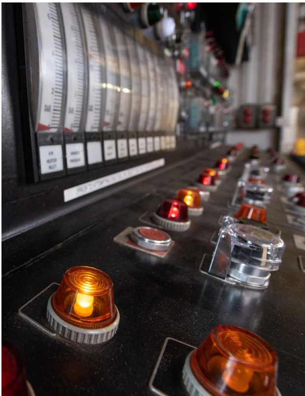
Parallel positioning boiler controls can save 5% to 7% of fuel consumption.
