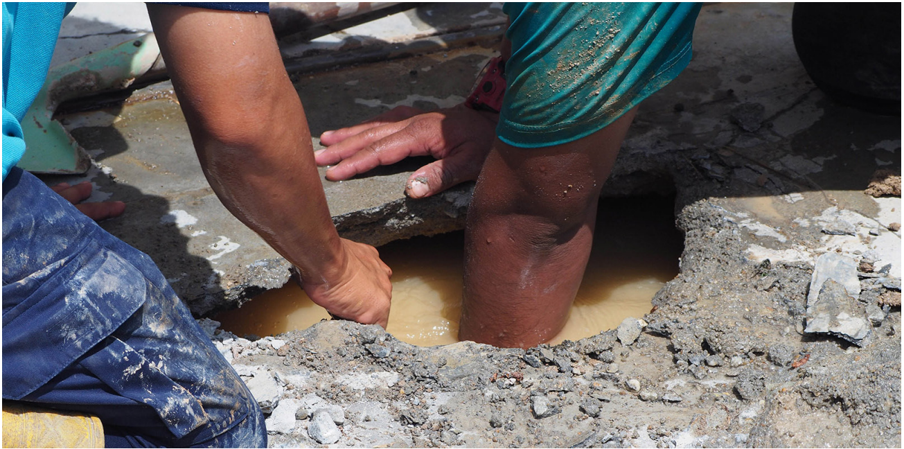
An indicator of a potential leak is a heaving or cracked area of pavement.
