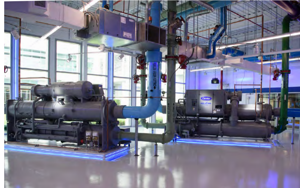
Two Carrier AquaEdge 23XRV Chillers at the UTC Center for Intelligent Buildings, Palm Beach Gardens, Florida.
