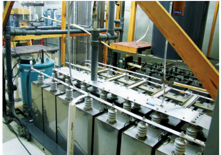
Lightning test facility
